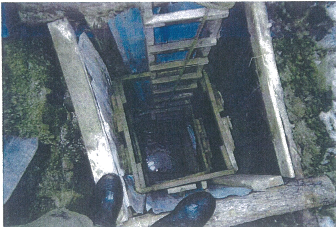
THAWED WET AT BOTTOM CC-4 (FLOODING) MARCH 27, 2015
