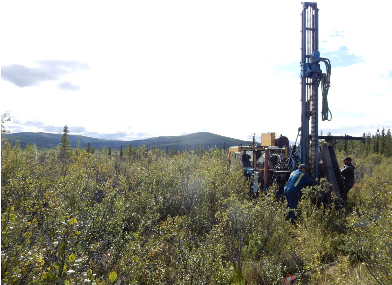
Plate 3 - Sylvain Fleurant drilling on the GRGP property using a track-mounted six-inch auger drill in August, 2020.
