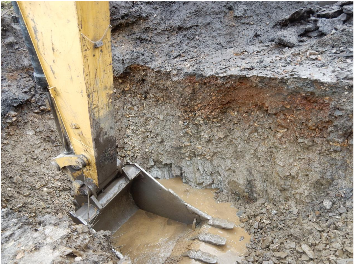
Figure 19 - Test pit 2020-01 was excavated on June 11, 2020 to bedrock a depth of approximately 4 metres from surface, just upstream of an earlier test pit (2019-10) which was dug in 2019. Angular bedrock can be seen in the photo below a sandy cobble gravel. Bedrock was dipping towards the left side of the photo implying that the deepest part of the channel was not sampled.
