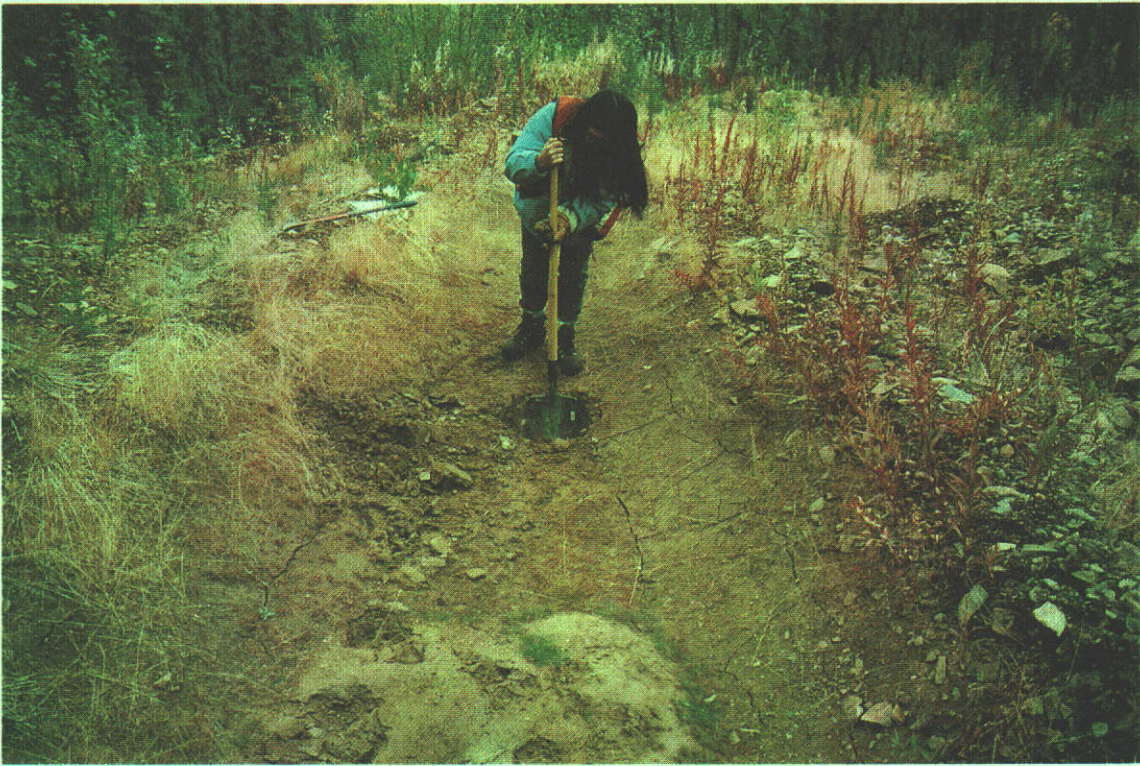
Plate 3-6 Trench N3. Fine-grained material accumulates at the floor and lower end of the trench.
