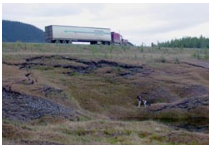
Figure 9. Debris slide related to growth of a thermokarst depression adjacent to the Alaska Highway near Dry Creek (see Figure 8). Thermokarst activity was initiated after overlying vegetation and gravel was removed by aggregate mining for highway construction.
