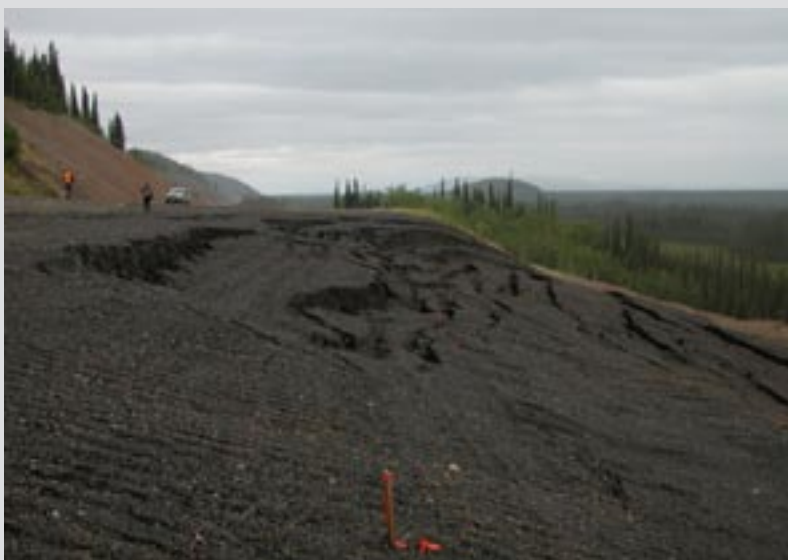
Figure I. Initiation area of failure caused by subsidence due to permafrost thaw at the base of the slope. Note car parked on Alaska Highway shoulder for scale. View looking southeast.
