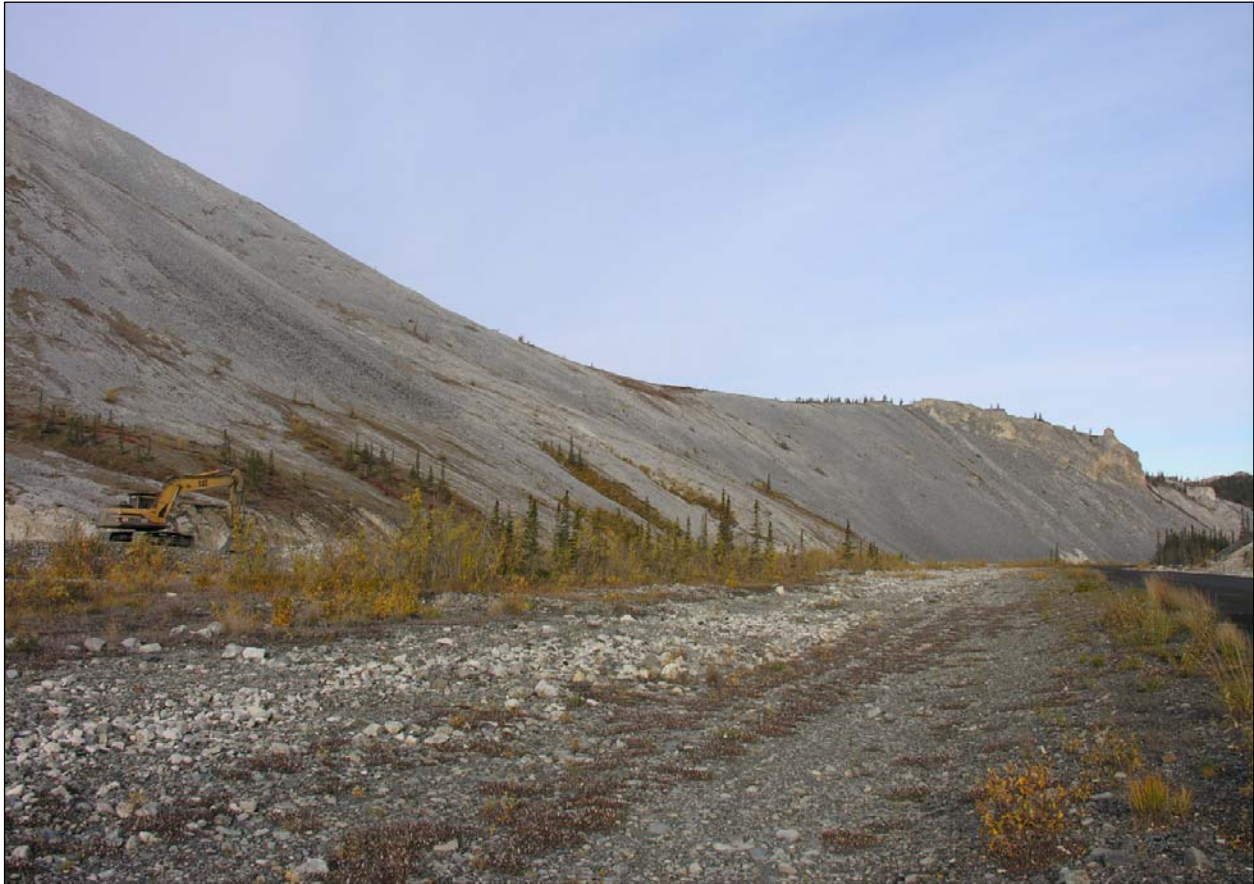
Figure 29. This large hoe is repairing a levee to restrict floods from damaging the highway (Km 156). Also note dark shale used to surface this stretch of highway.
