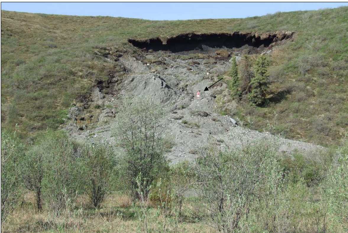
Figure 23. Slope failure cause by melting permafrost. Person for scale.
