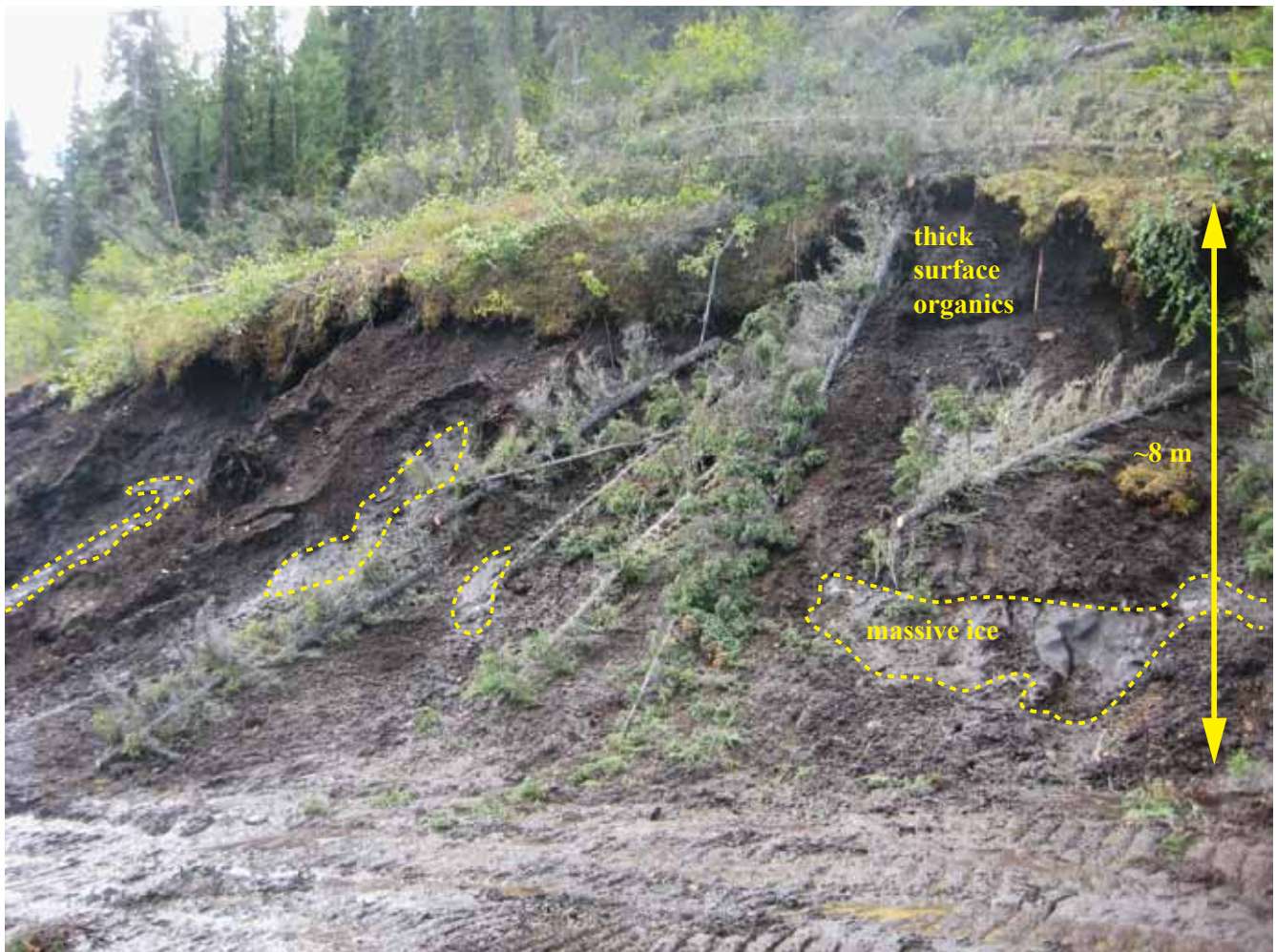
Figure 10. Fresh road cut into permafrost on east-facing valley side of lower Britannia Creek. Note thick, mossy surface organic layer and massive ice bodies.
