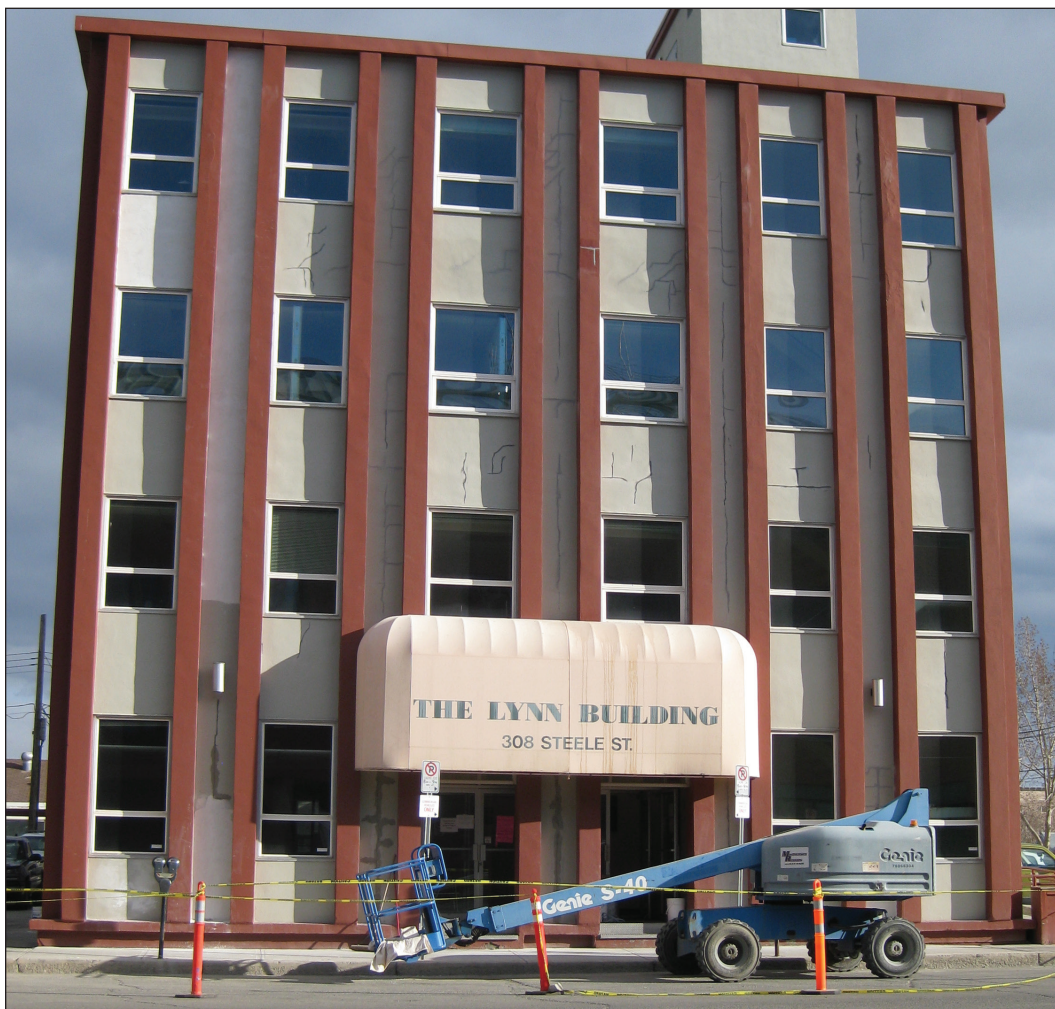
Figure 47. Repairing cracks on the exterior of a downtown Whitehorse building, following the May 1, 2017 earthquake (May 9, 2017 photo).
