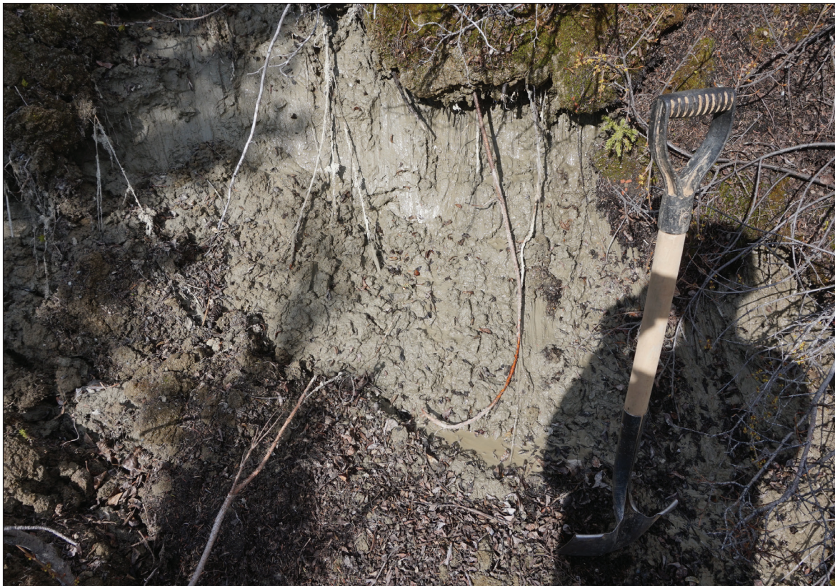
Figure 37. Tension crack in saturated ground adjacent to Drury Street slide source zone (May 26, 2022; Jeff Bond photo).
