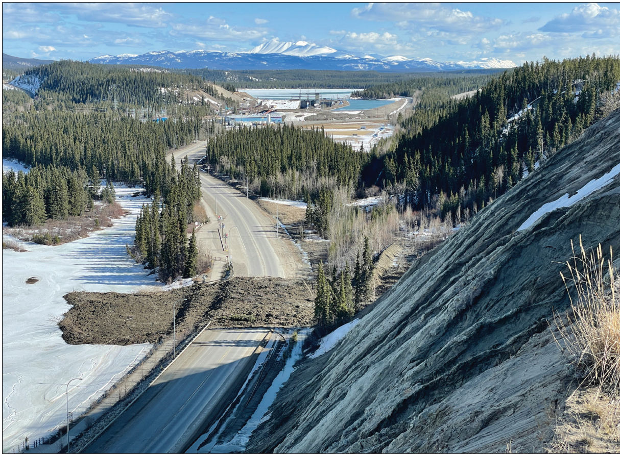
Figure 34. Slide debris extending across Robert Service Way and Millenium Trail on April 30, 2022.
