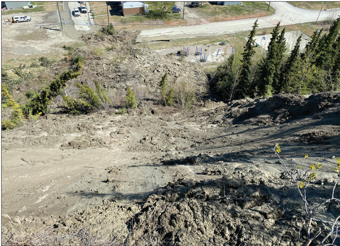
Figure 41. View looking down Jeckell Street slide from the headscarp (May 28, 2022 photo).
