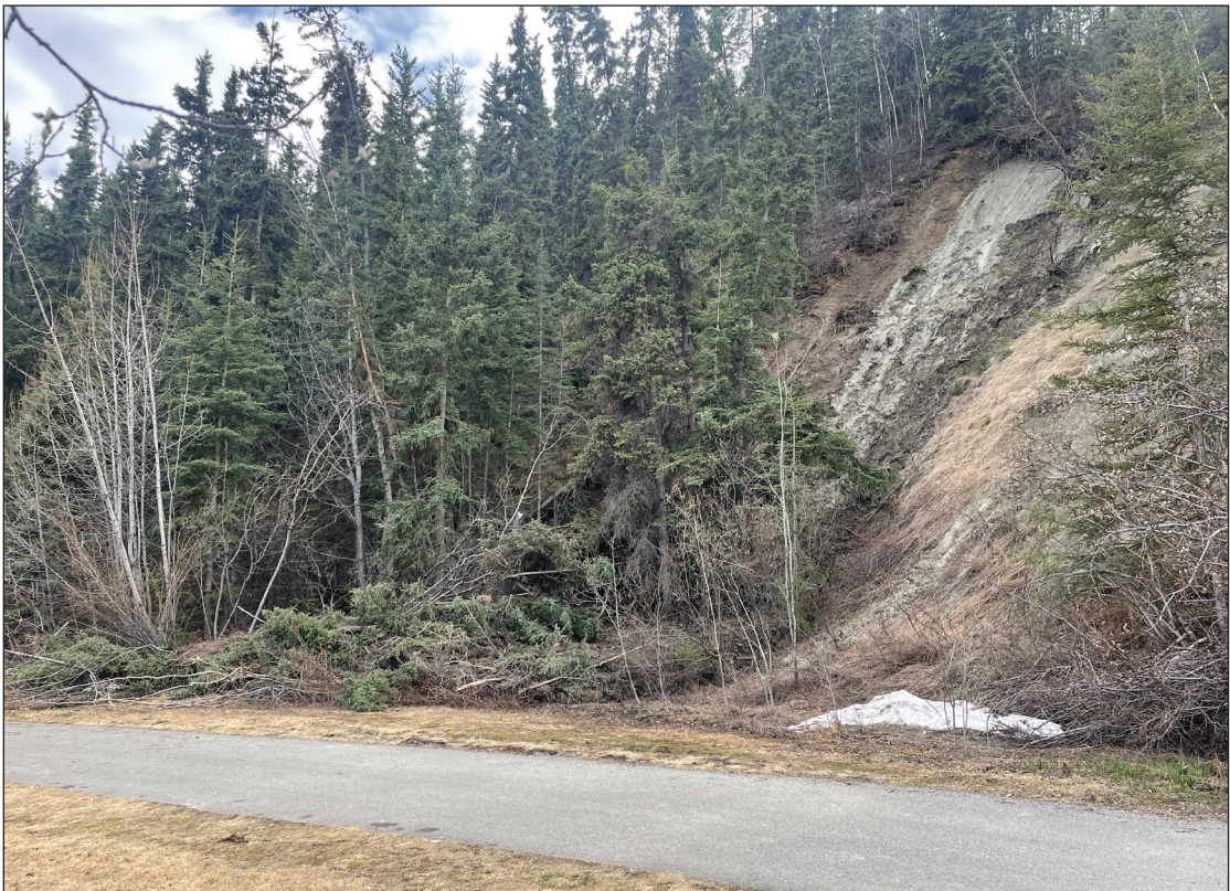
Figure 40. A small precursor slide occurred on May 18, 2022 on the north flank of the May 27, 2022 Wood Street slide.
