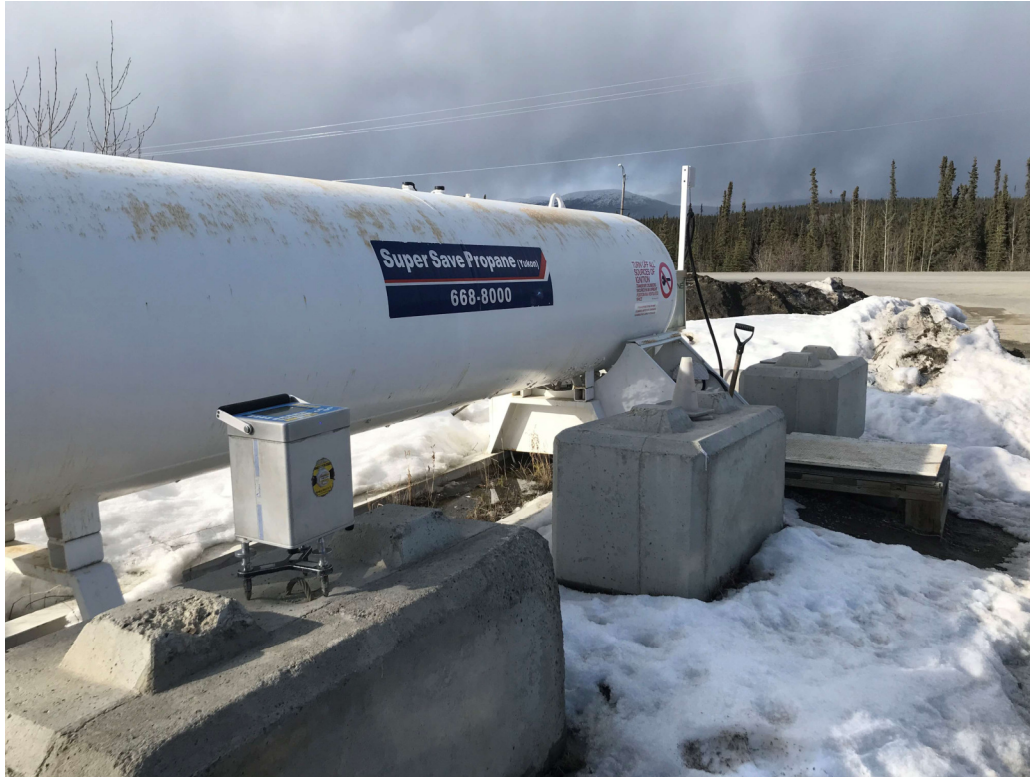
Figure 10: Control station at Nisutlin Trading Post in April 2022 (Station 8880).
