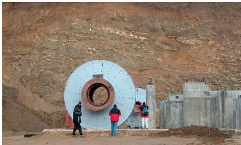
Figure 9. Semi-autogenous grinding mill, ball mill and mill footings at the Minto mine property.
