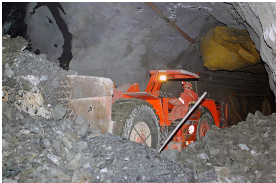
Figure 7. Advancing the underground workings at the Wolverine property. (Photo credit: Yukon Zinc)
