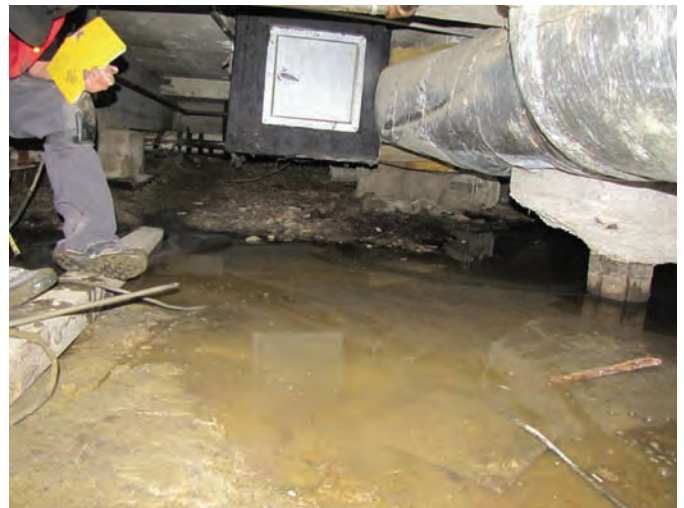
Figure 5. Water in crawl space beneath Palace Grand Theatre, July 25, 2010; note the exposed piling below concrete pad indicating the presence of ground surface subsidence.
