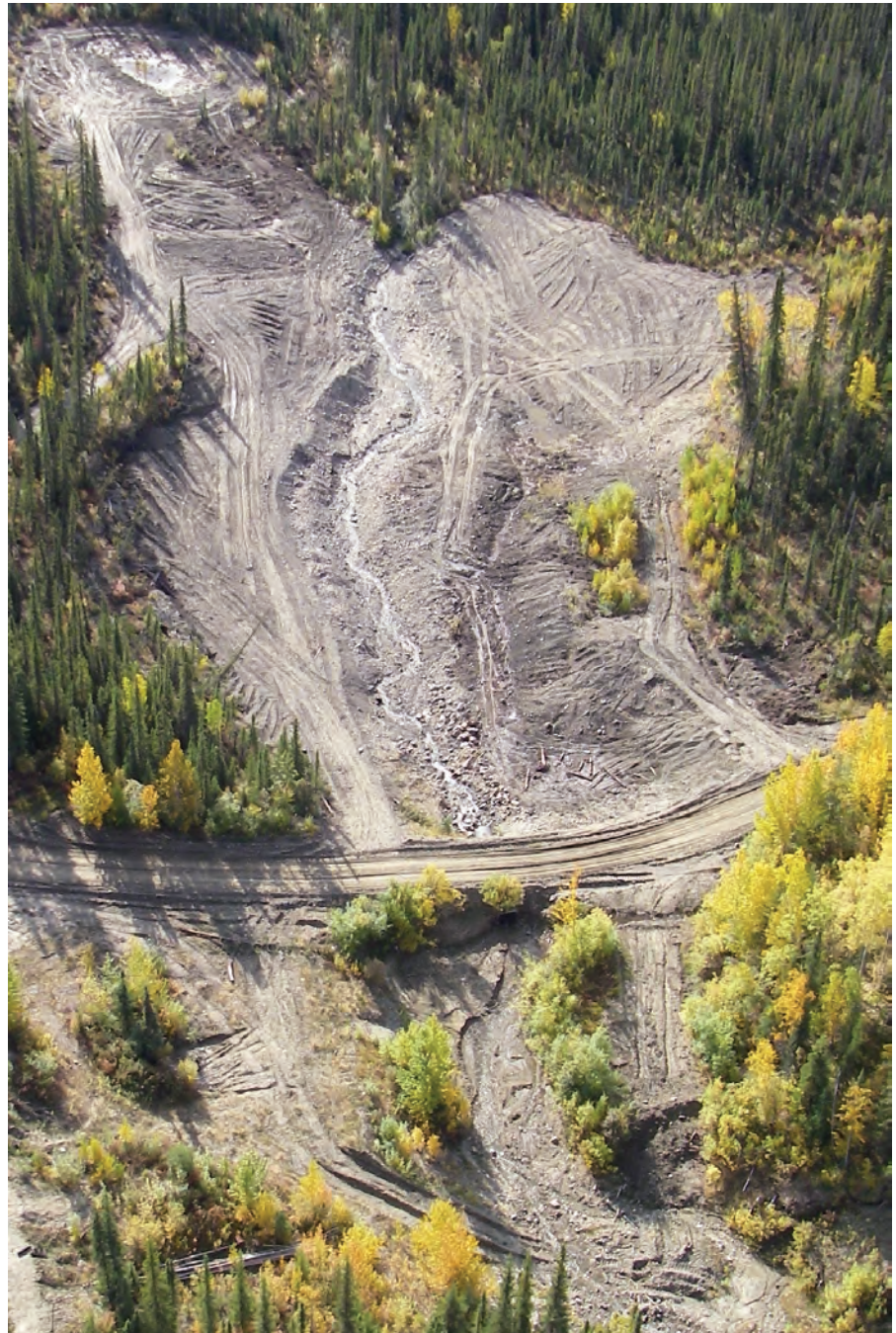
Figure 2. Sloped, contoured and scarified area along Haggart Creek Road, near Mayo. Reclaimed area was covered in fines to enhance re-vegetation.
