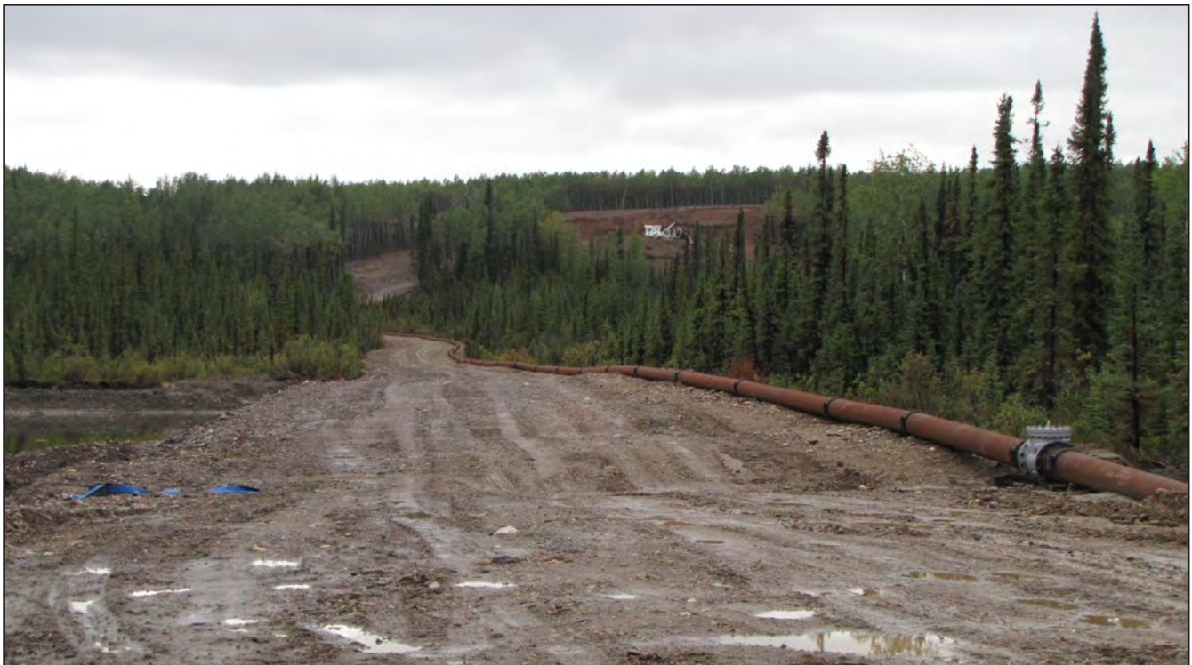
A view of the water line constructed from Clear Creek. The Big Alex bench and the wash plant is visible in the distance.
