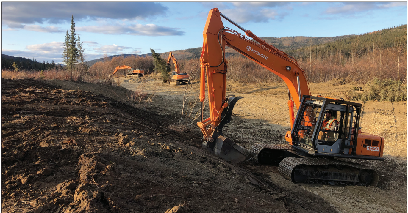
Figure 5. A view of the new Sulphur Creek channel being constructed on Yukon Heliski's ground in partnership with RESOLVE, Tiffany & Co., and Apple. Photo courtesy of Pete Wright.
