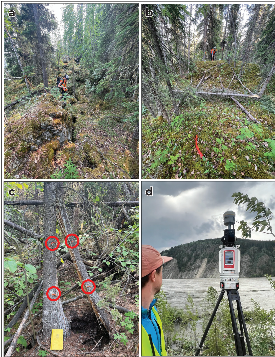
Figure 5. (a) Tension crack near TCMS station 2. Recent movement is shown by the gap between the rock and moss growth. (b) TCMS station 6. (c) Split tree near TCMS 8 with nail monitoring installed. This crack opened 2.2 cm and 3.3 cm between June and September 2022 at the upper and lower nail sets respectively. (d) Terrestrial lidar scanner with the Sunnydale slide in the background across the Yukon river, note the shallow landslide directly left of the scanner.
