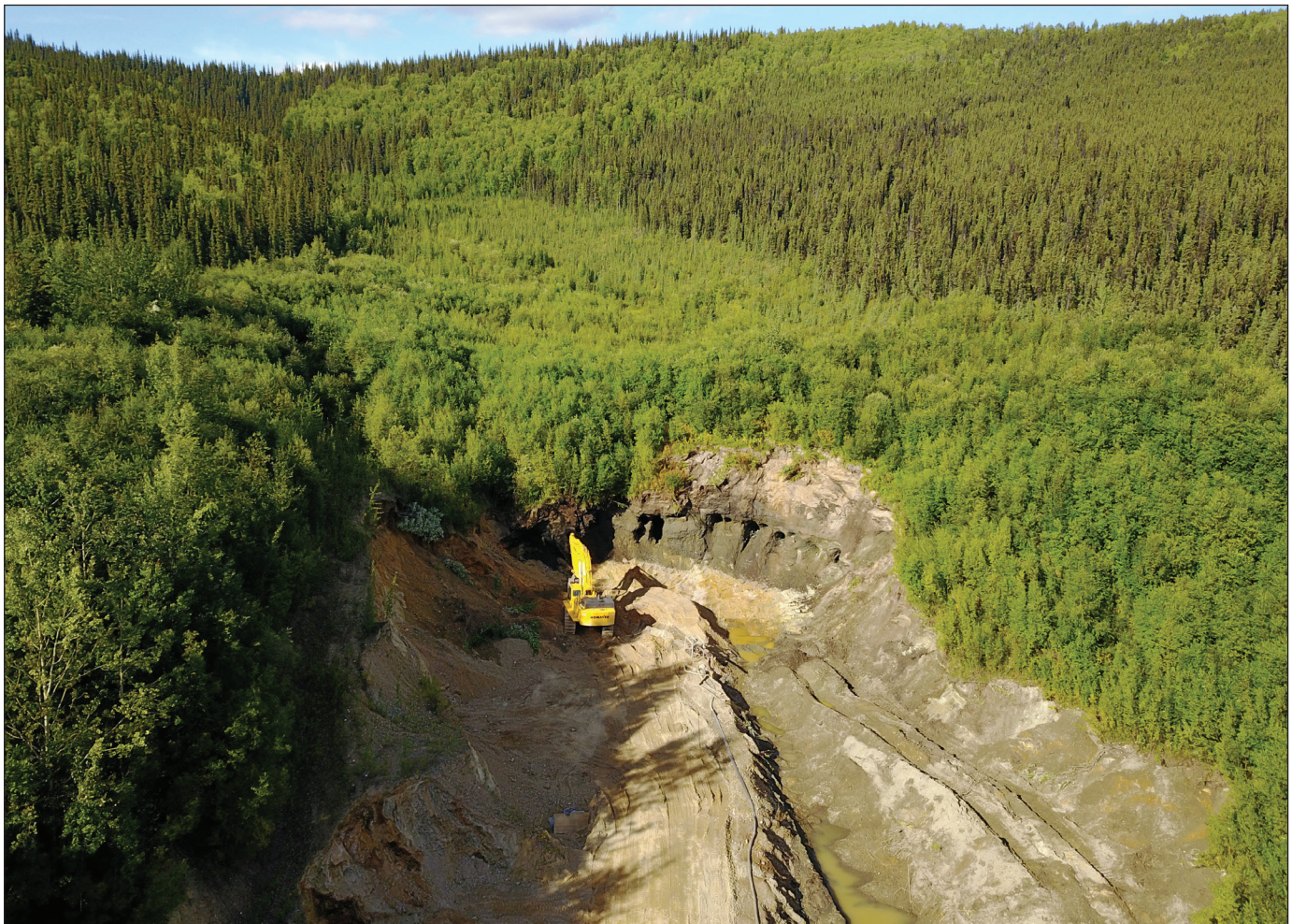
Figure 4. Drone image looking up Green Gulch, with Lucky Dog Mining's active cut in the foreground.
