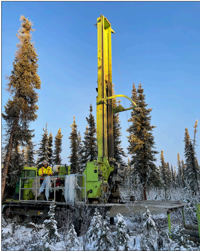
Figure 2. Northern Sonic Drilling and Consulting’s sonic drill at site YGS_BeaverCreek_BH4 in Beaver Creek.
