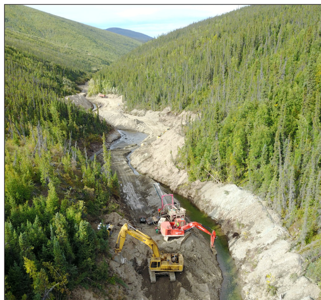
Figure 11. Aerial view of Moose Creek; a John Deere 992 excavator (yellow) gives perspective of the narrow nature of the creek.
